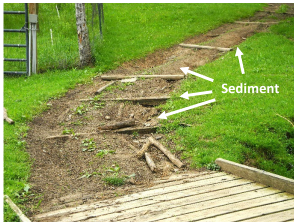
Lower 20% Grade with Significant Erosion
