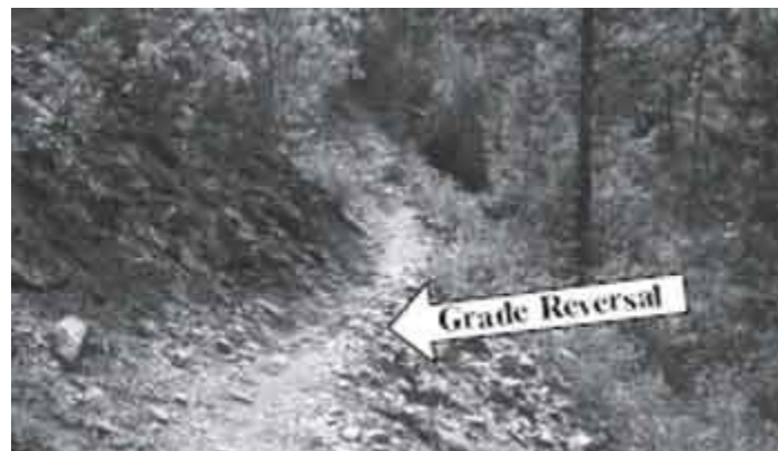
Figure 11 – Grade reversals are much more effective than waterbars and require less maintenance. Grade reversals with outsloped tread are the drainage structure of choice.
