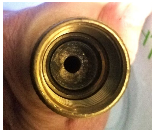
Corroded drain hose fitting
